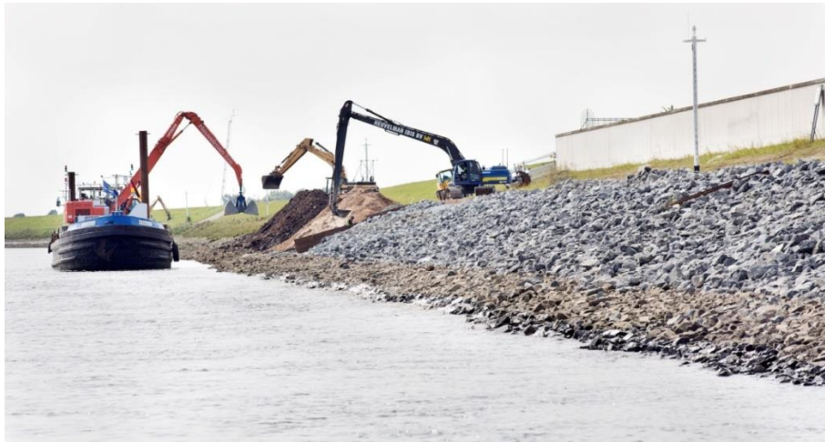
Figure 1: Construction of an embankment from aggregates; armourstone (top layer) and grain filters
